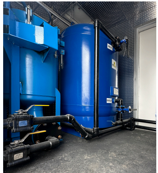
Three part water filtration system and holding tanks for tank car cleaning
